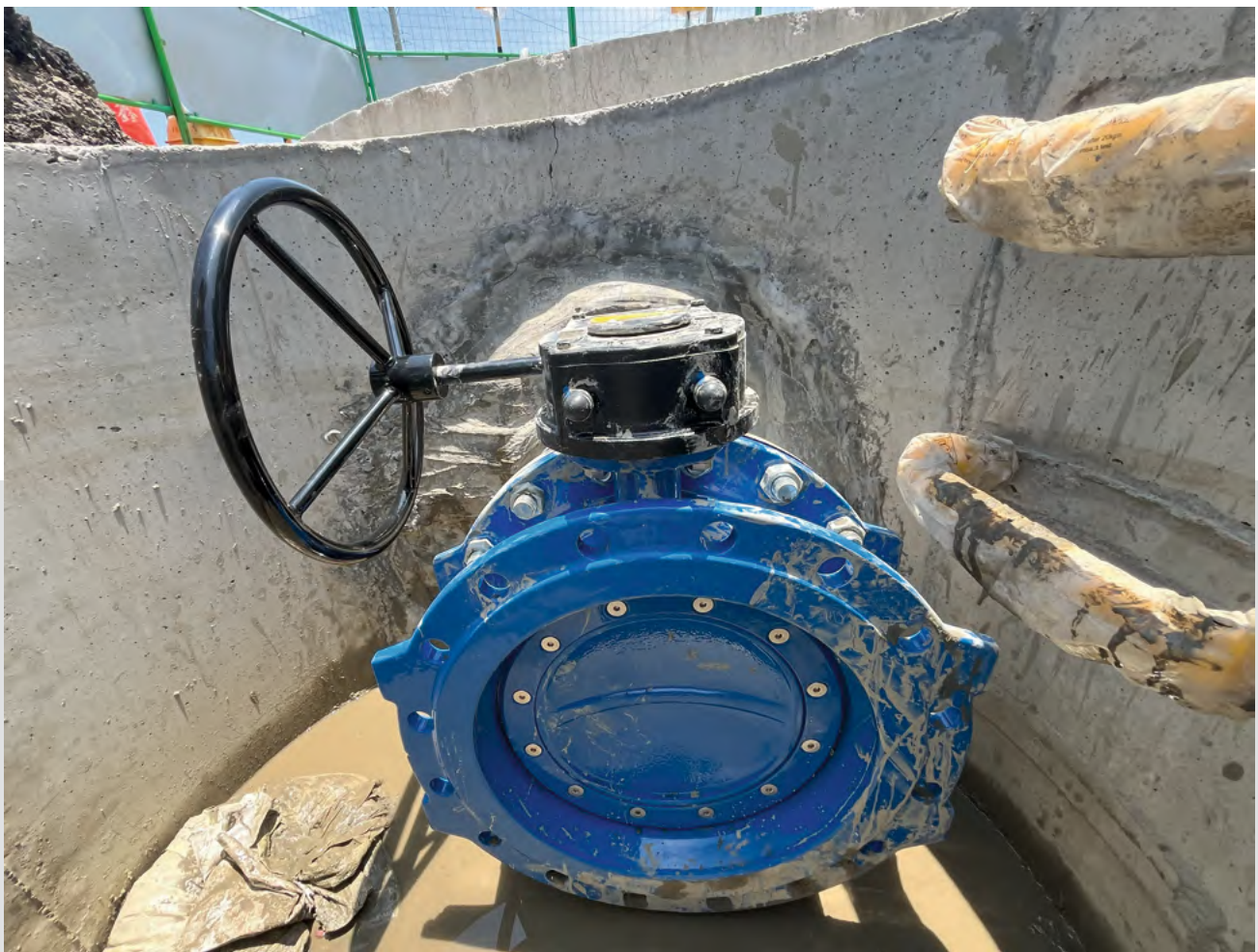
Butterfly valve installed
