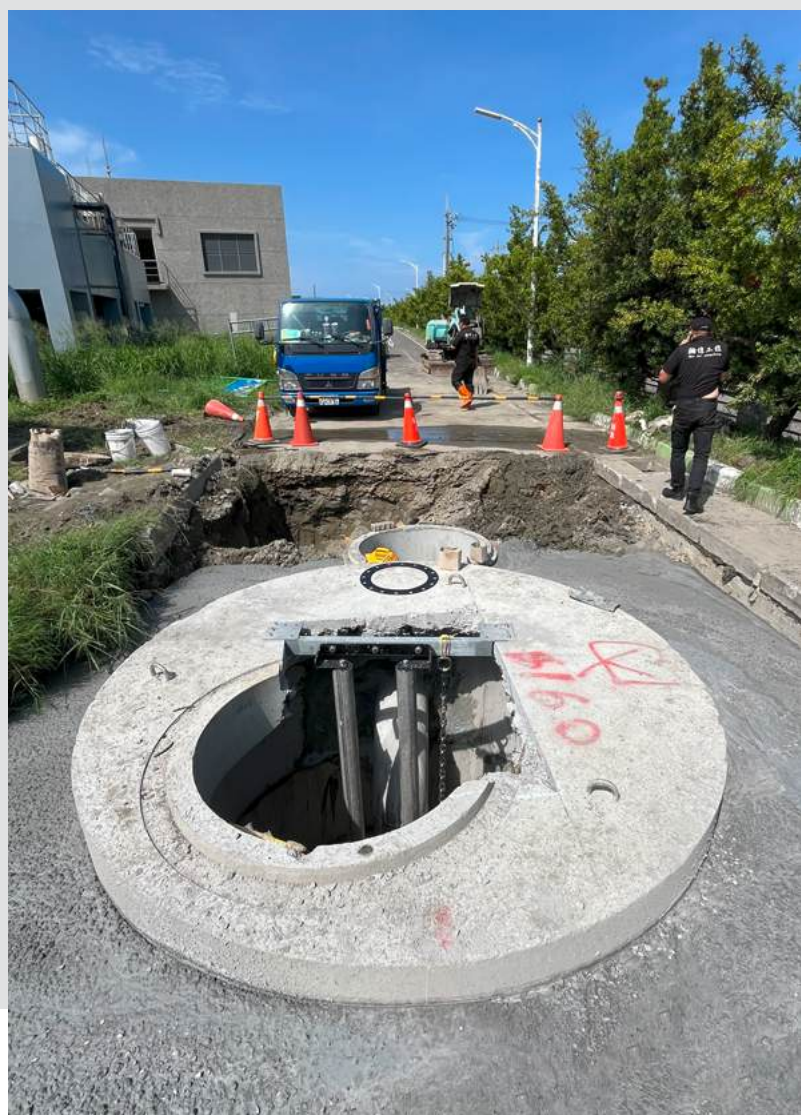
Valve installation location
